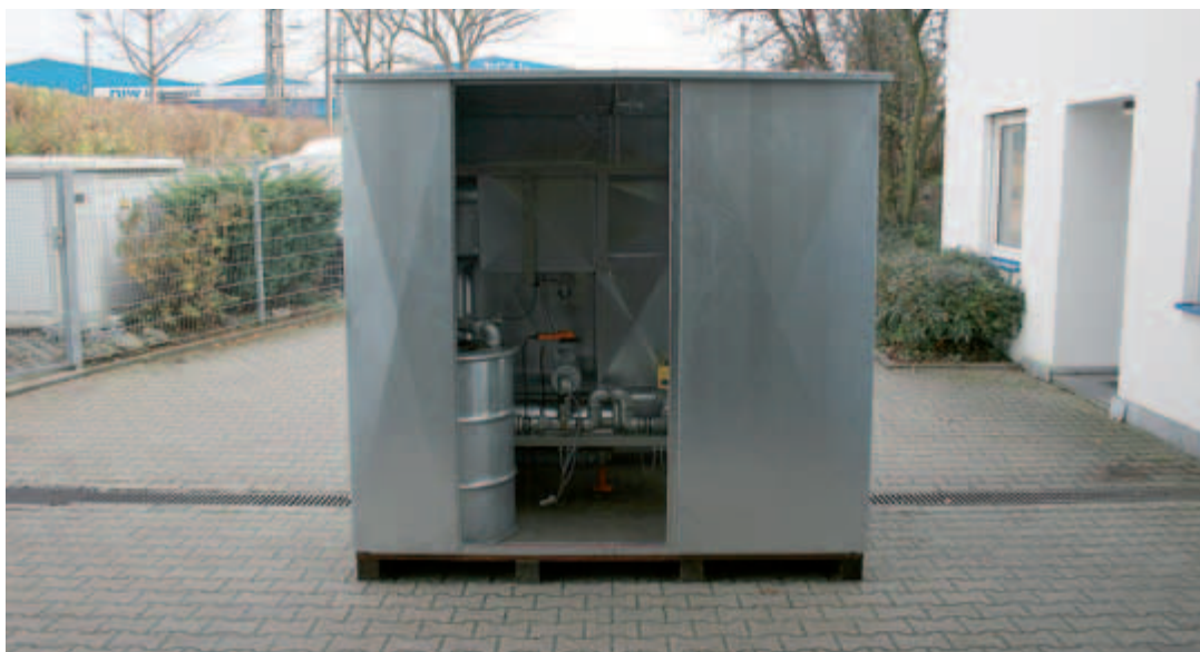
CATOX 100 combined with cleaning of groundwater
