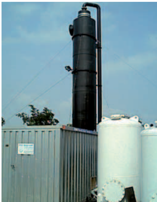
Tower air stripper TS 10 with downstream activated carbon filter units and an equipment container
