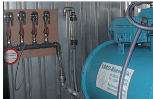
VAK 100 use for 4 extraction wells
