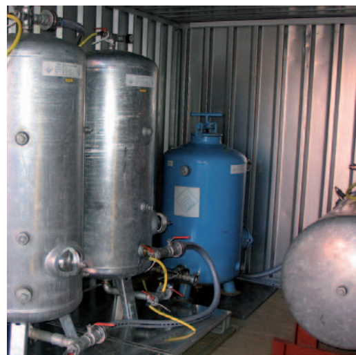
AKA 7 fixed in a closed equipment container
