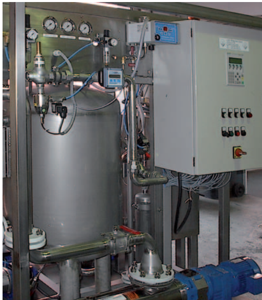
Example of a membrane plant
